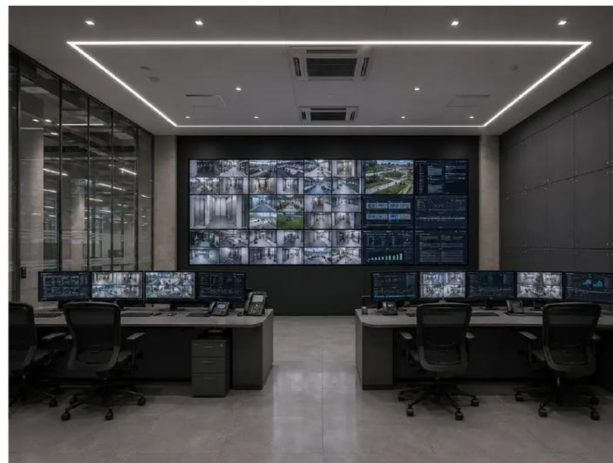
COMMAND ROOM • SURVEILLANCE, ACCESS, FIRE AND BUILDING SERVICES RESOLVED ONTO ONE WALL
